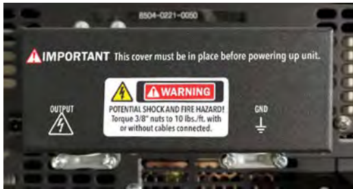
Figure 3.3 – Output Safety Cover
