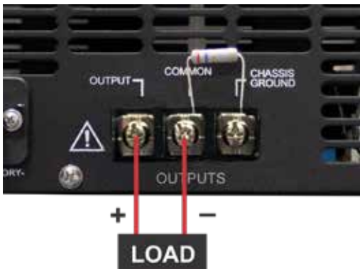
Figure 4.2 – Connecting the Load
