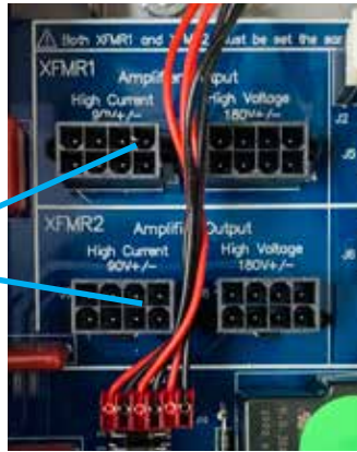
Figure 6.9 – Location of Amplifier High-Voltage Transformer Sockets
