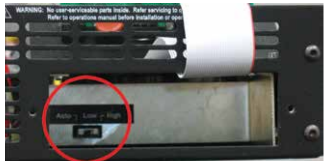
Figure 6.12 – Bi-Level Power Switch Location
