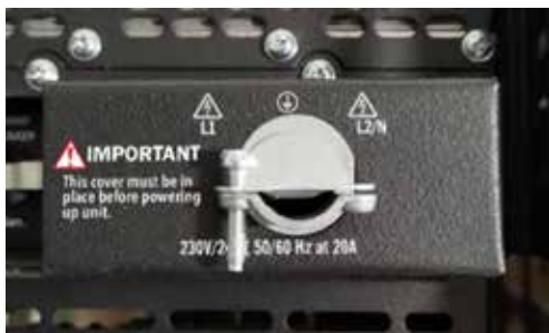
Figure 3.8 – AC Inlet Safety Cover
