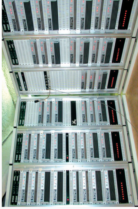
Amp room at Sooyoung Ro Church in Pusan, South Korea.
