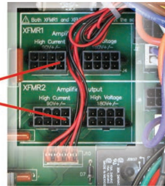
Figure 5.10 – Location of Amplifier High-Voltage Transformer Sockets
