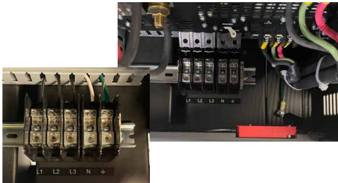
Figure 3.5 – Location of AC Mains Barrier Strip with labeling detail (inset)
